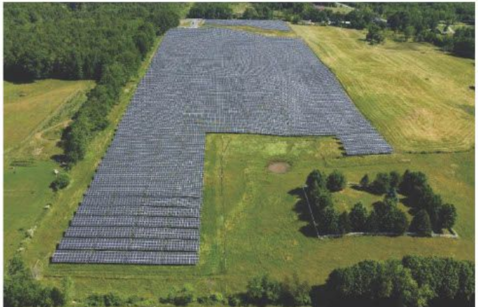
A 7.3-MW community solar project in Farmingdale, Maine, owned by Nautilus Solar Energy.
